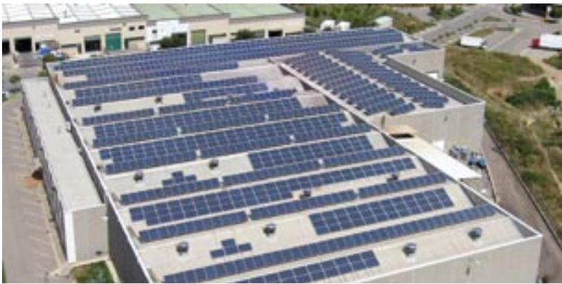
6,000 m 2 WATT SOLAR industrial rooftop installation in Osona. Capacity: 233.20 kWp (1,166 modules)
